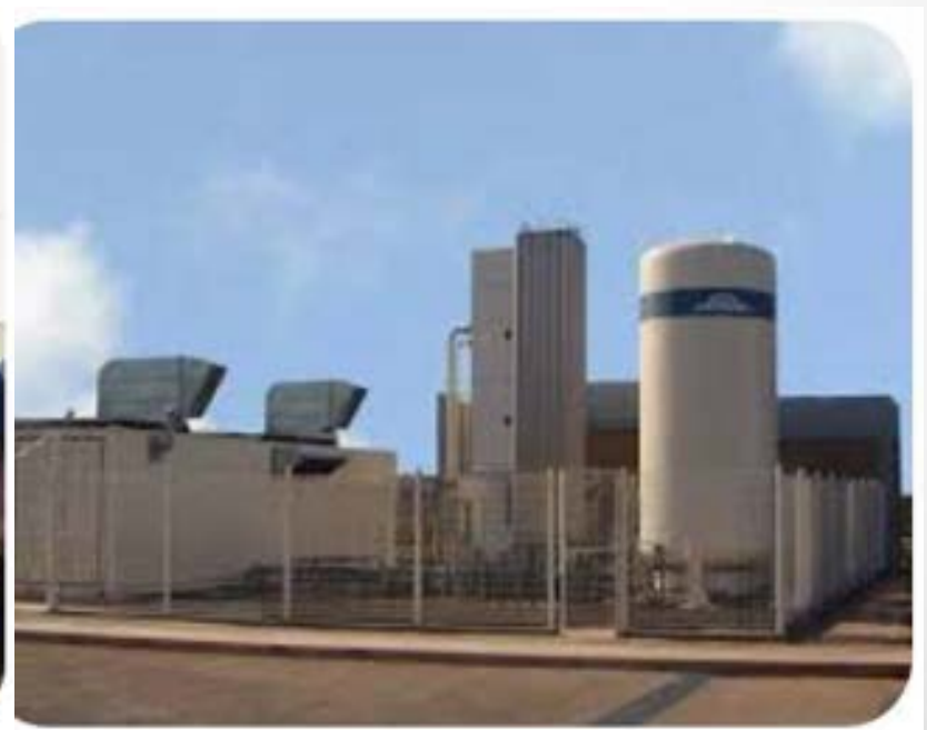
Oxygen generation station
