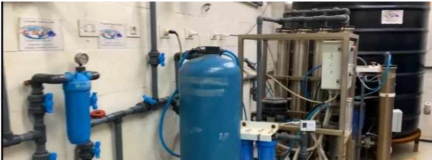
Mobile water treatment unit at the College of Earth Sciences
